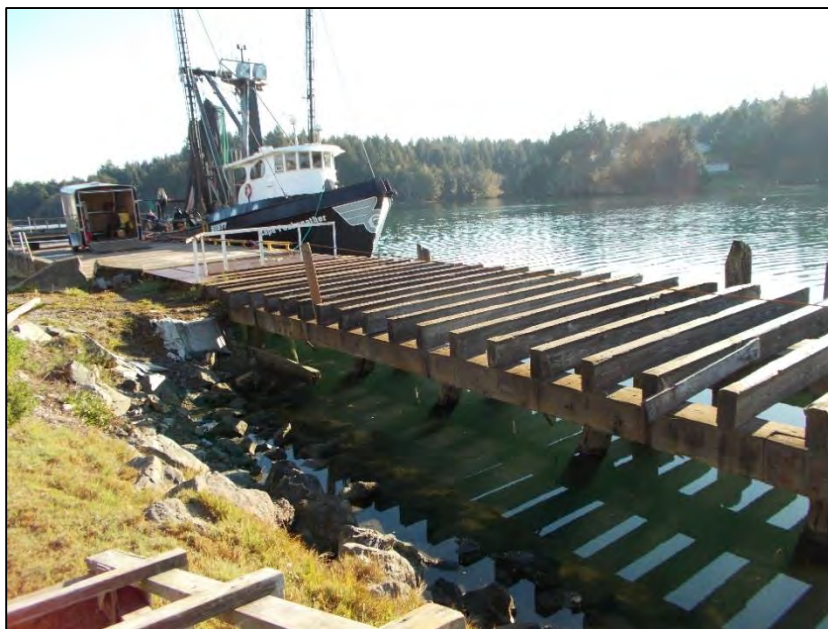
Photo 17. Unusable work docks
