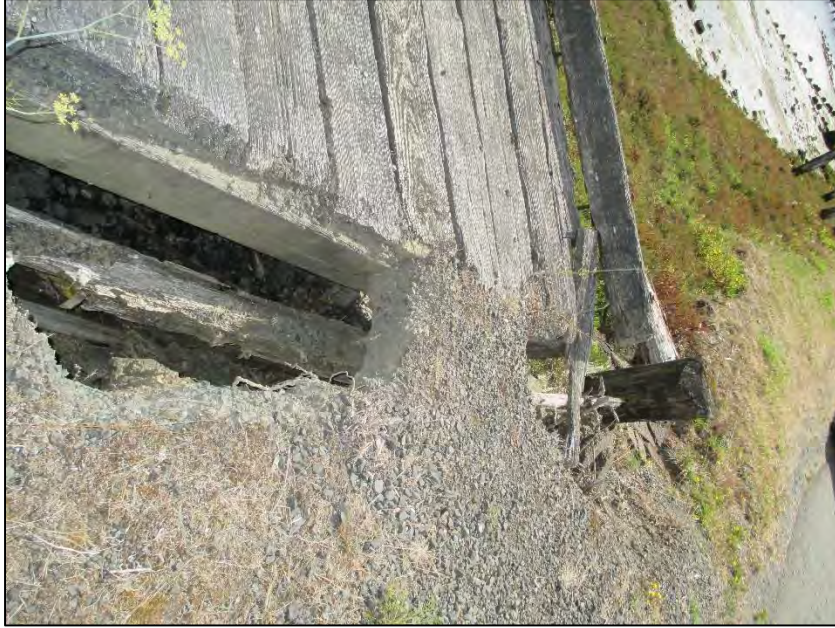
Photo 33. Gap at abutment
