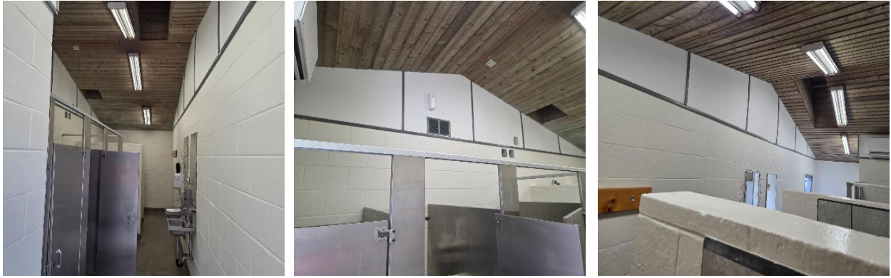
The finished look of the men's restroom and showers at the RV Park.
