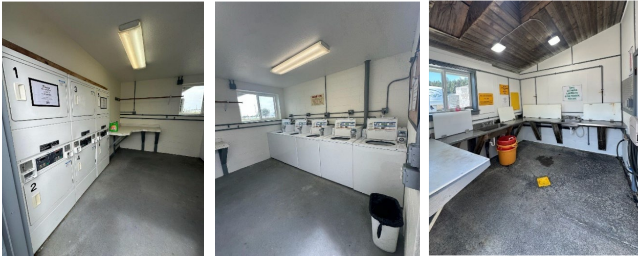
Fresh paint on the walls of the RV Park laundry room and the crab/fish cleaning room.
