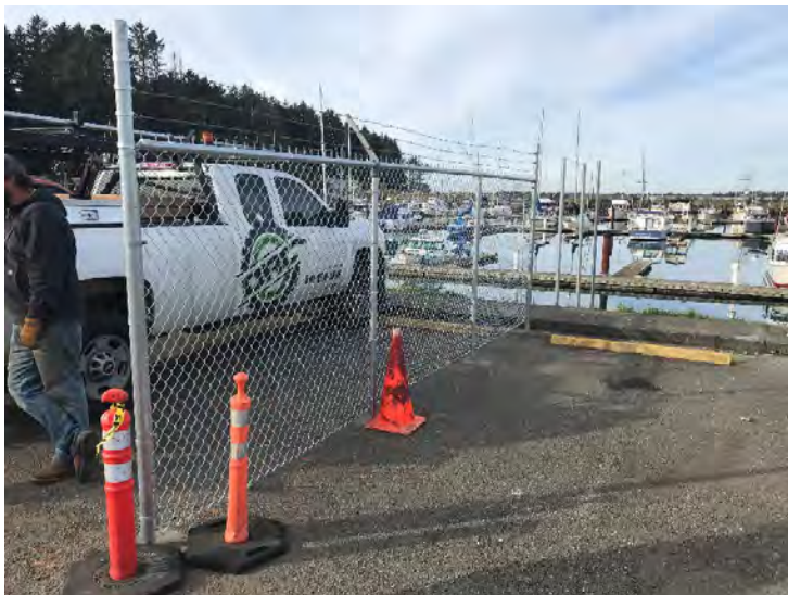
Local Contractor from Darrel Rogers Construction finishes up the barbed wire on top of the fence at I-Dock.
