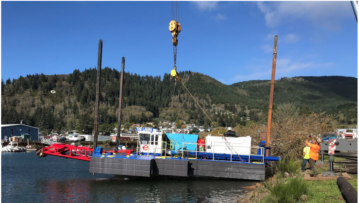
Forslund Crane Services launches The Laura, the dredge owned by the State of Oregon using their 350-ton crane.
