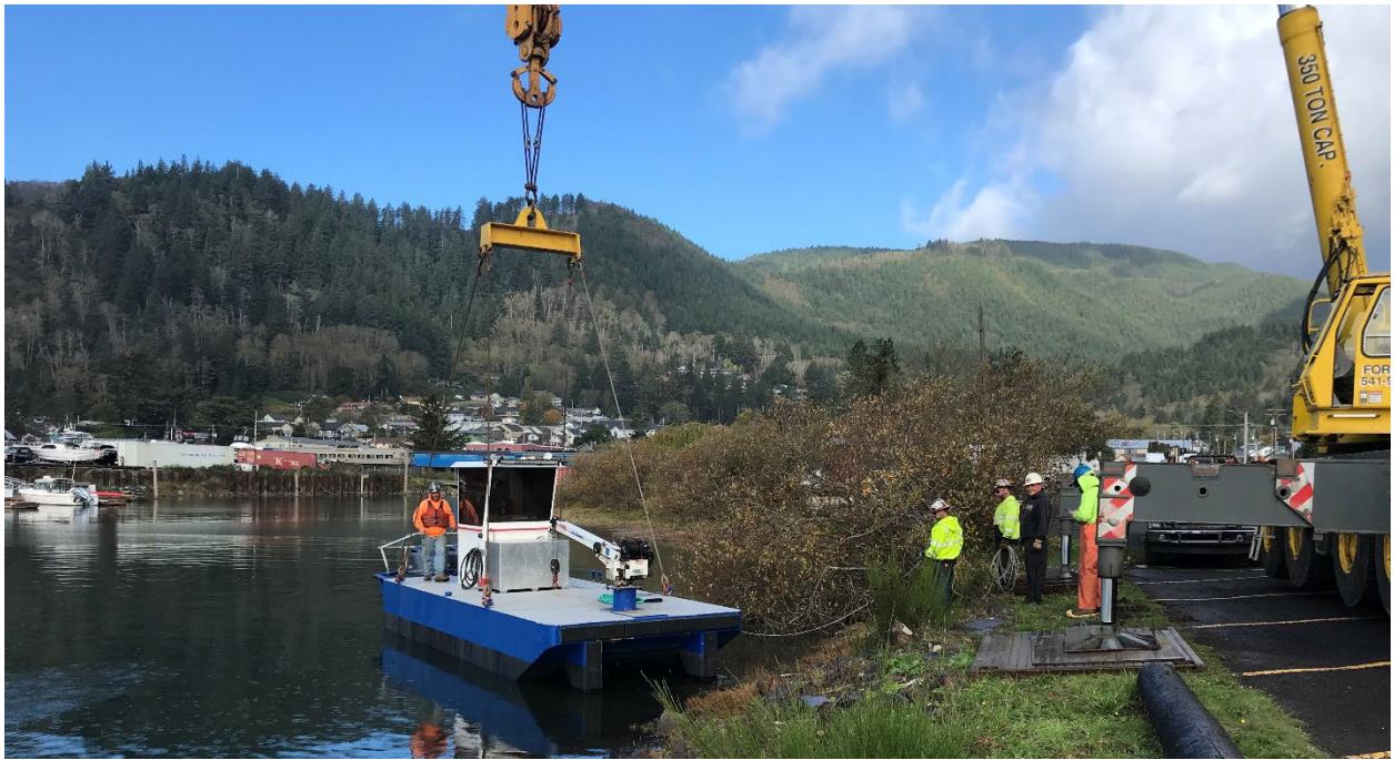
David Stevenson, Maintenance Apprentice II, boards the support vessel Ms. SoCo after she was lifted from her trailer and placed into the water by Forslund Crane Services.
